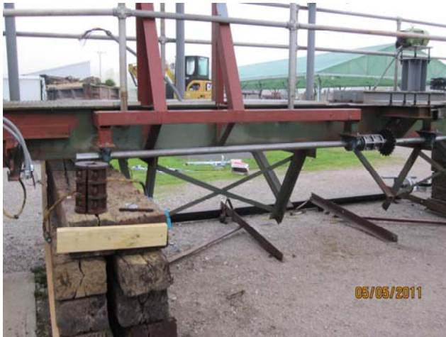
All new Drive System & Electrical Components
